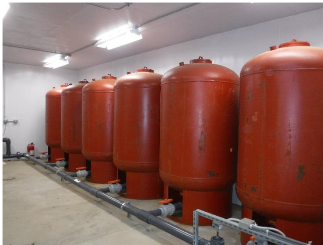
Figure 4: Water Storage Tanks
