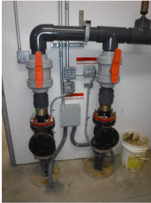
Figure 3: Raw Water Intake
