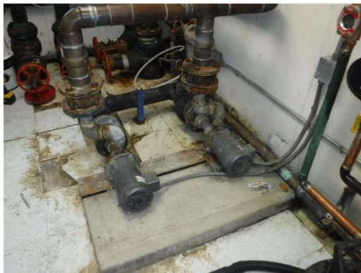
Figure 12: Water Circulation Pumps
