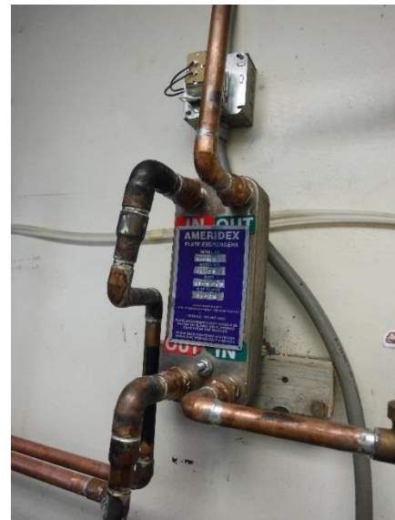
Figure 13: New Water Circulation Heat-Add Heat Exchanger
