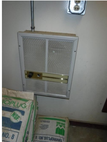
Figure 6: Generator Room Electric Heater
