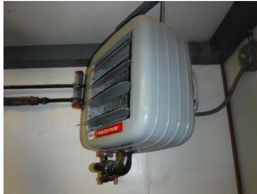
Figure 9: Water Treatment Plant Unit Heater
