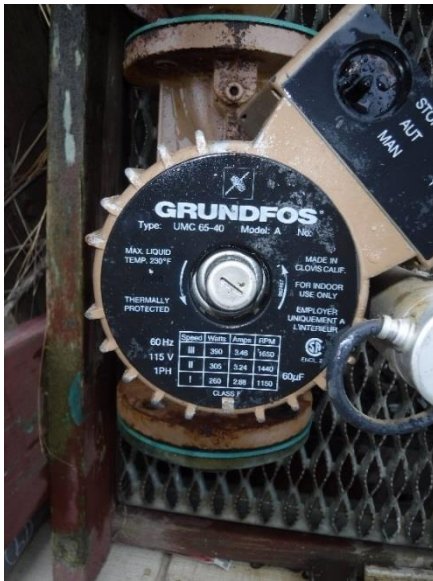
Figure 10: Old Glycol Circulation Pumps
