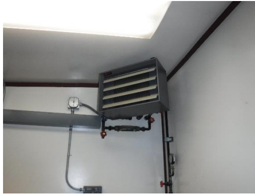
Figure 8: Generator Room Unit Heater
