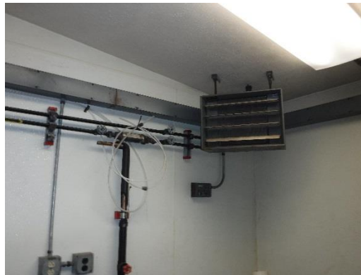
Figure 7: Storage Room Unit Heater
