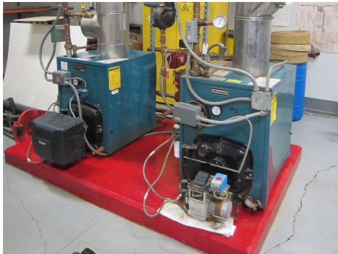
Figure 4: Boilers in the water plant.
