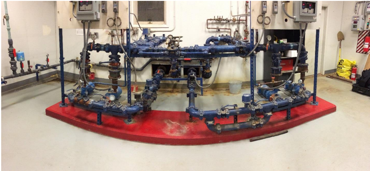
Figure 2: Main room in New Stuyahok Water Plant
