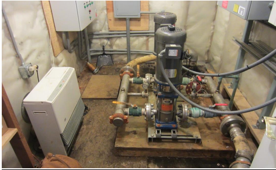
Figure 7: Inside the booster station, Monitor 422 on the left.
