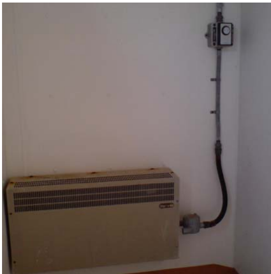
(Wet well heater)
