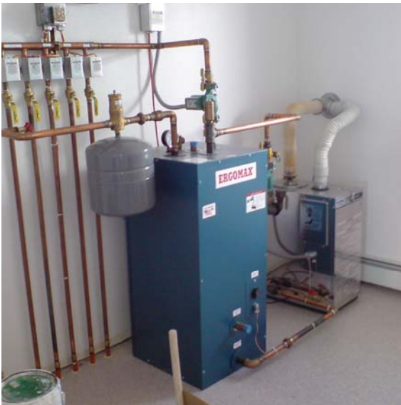
(Community Center Piping)
