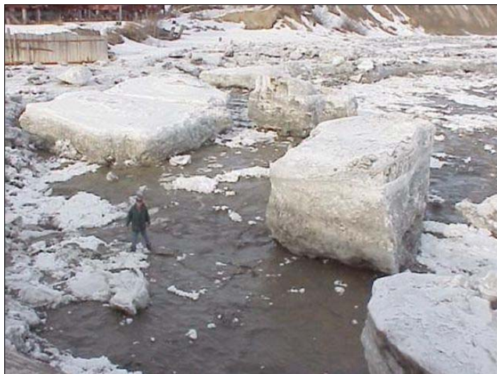
Large chunks of ice forms along the coastline during extreme cold temperatures. These large blocks of ice, called "anchor ice" holds sheets of ice in place while the Naknek River freezes over. Anchor ice has contributed to erosion of the shoreline and damage to docks and facilities in Naknek and South Naknek. Photo of Anton Littau and anchor ice, courtesy of Jeanine Littau, http://littau.net
