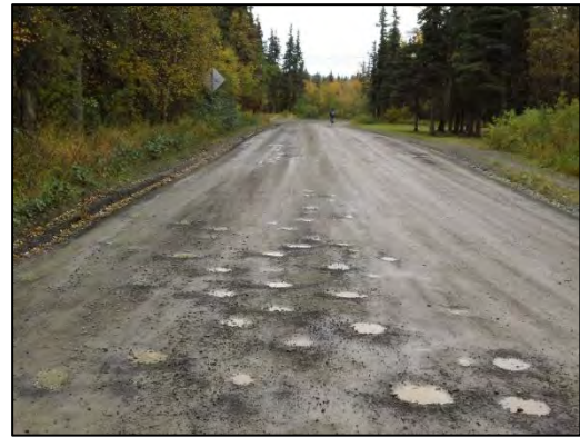
Potholes in Nerka Subdivision (Bristol, 2011)
