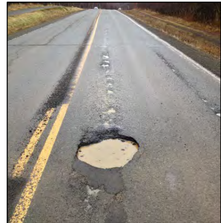
Pothole on Aleknagik Lake Road in Dillingham (KDLG, 2014)
