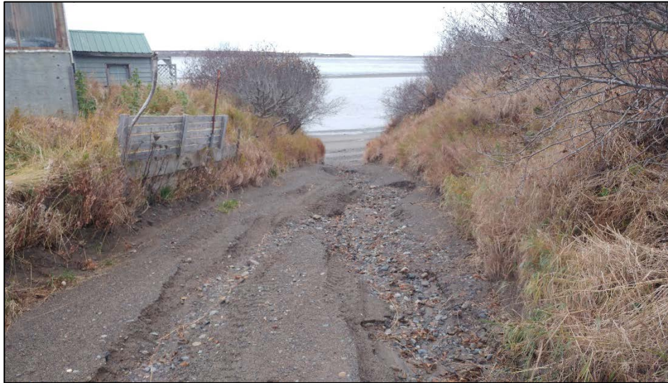
Photo 1 – Severe Erosion on Beach Access Road, October 2018
