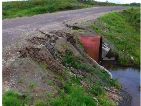
Eroding roadway embankment, 2016
