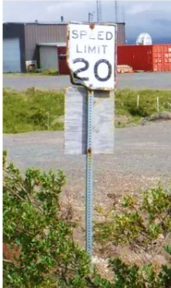
Damaged speed limit sign, 2016
