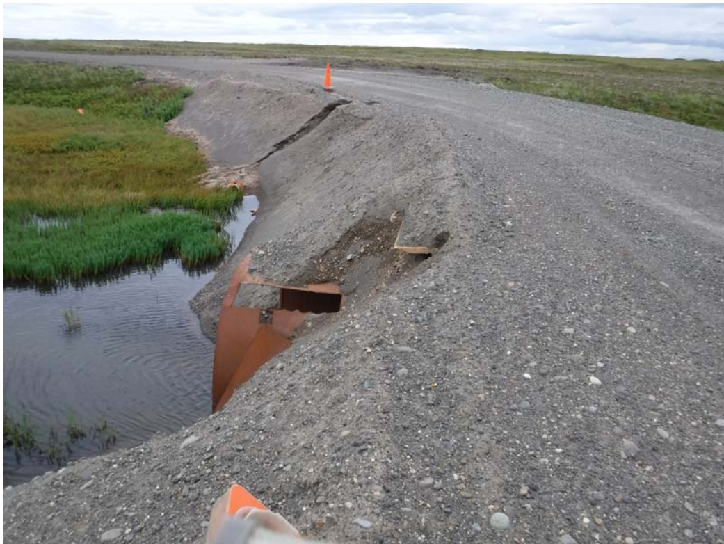
Photo 10 - Steep embankment erosion near culvert
