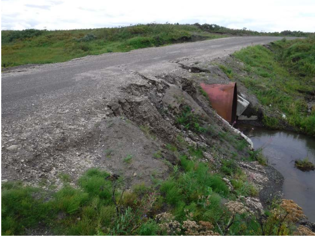
Photo 09 - Steep embankment erosion near culvert
