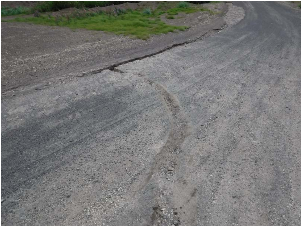
Photo 12 - Roadway erosion and poor drainage
