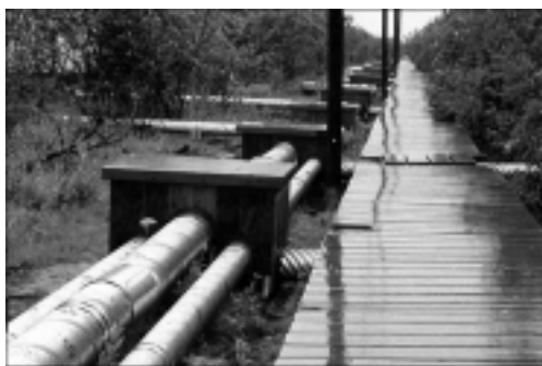
Piped water system.
