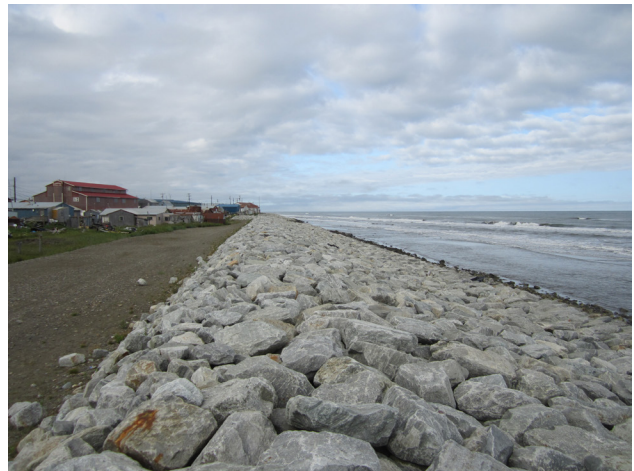
Figure 8. Shishmaref rock revetments. Photo taken August 2017.
