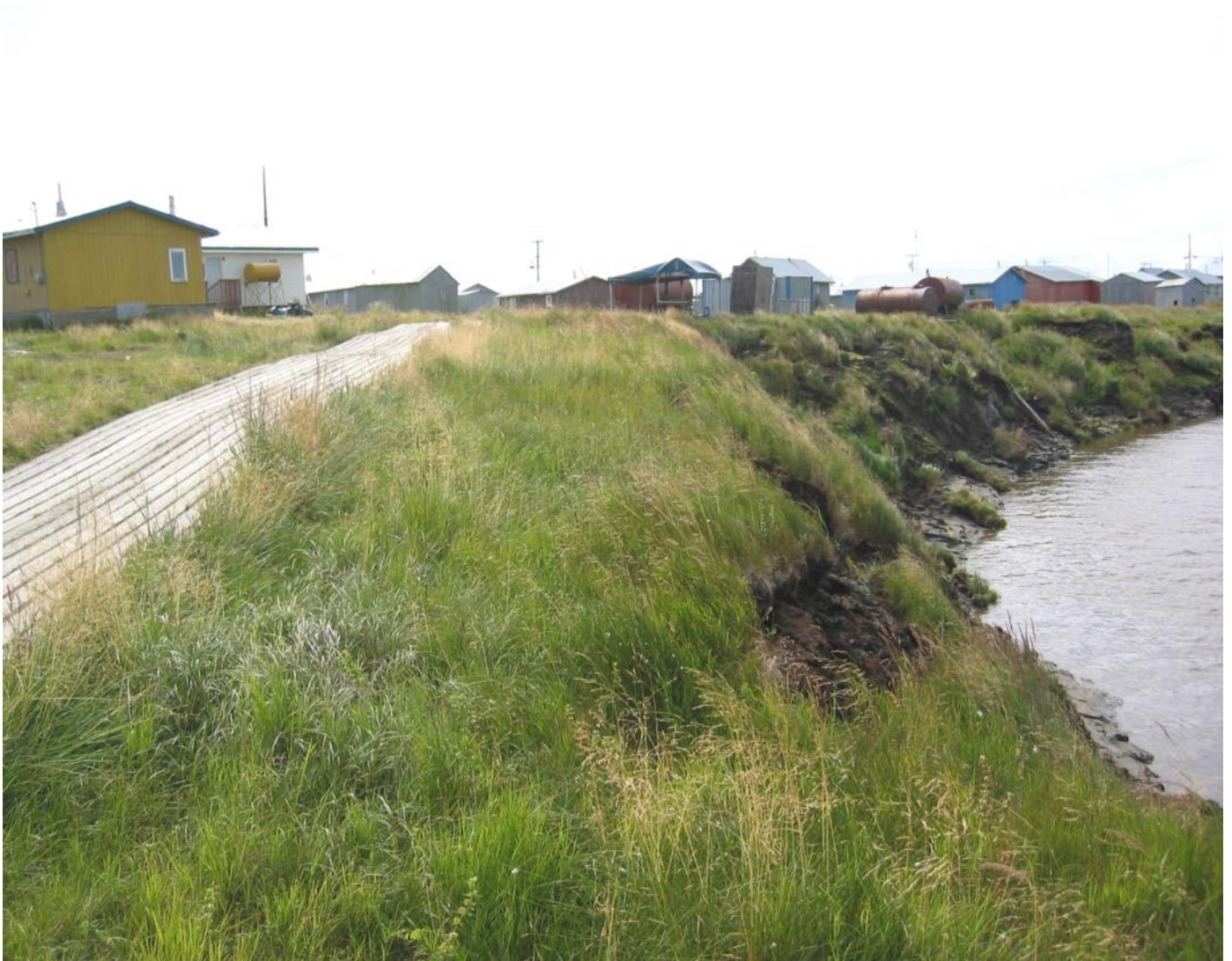
River bank erosion at Kongiganak, Alaska. Photo: DCRA/DCCED
