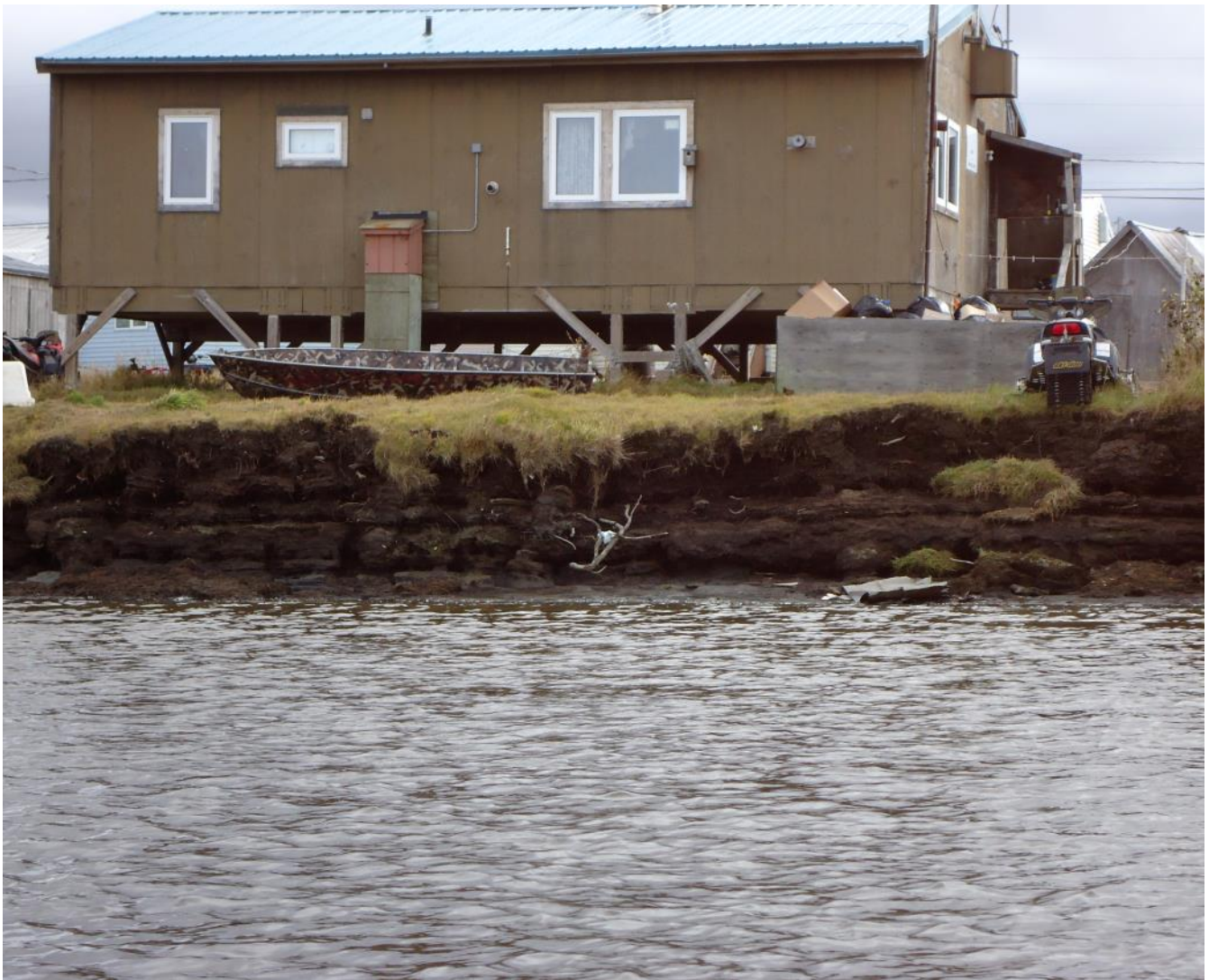
River bank erosion at Kotlik, Alaska. Photo: Lawrence Blood, DCCED/DCRA
