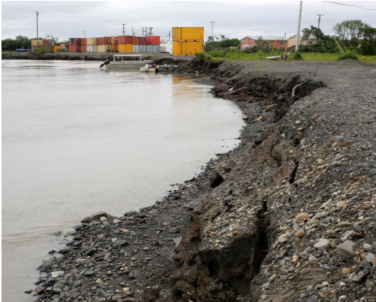
Heavily eroded bank of the Yukon River after severe 2013 flooding in the community of Alakanuk, Alaska. Photo: Federal Emergency Management Agency (FEMA).
